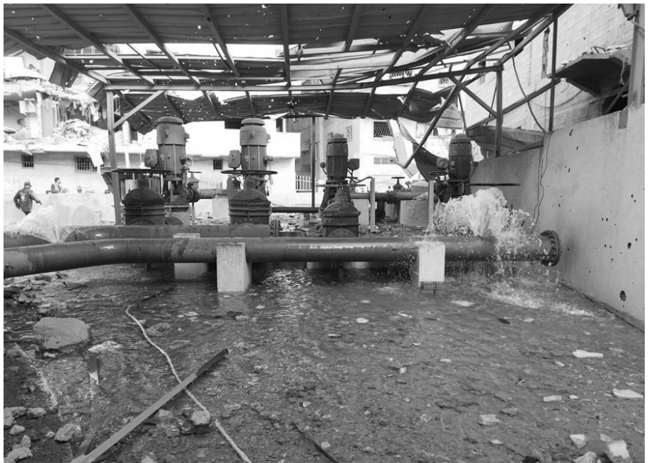
Extensive damage to a water tank in the Tal al-Hawa area, southwest of Gaza City, following Israeli shelling, Source: Gaza Municipality on Facebook - May 12, 2024
