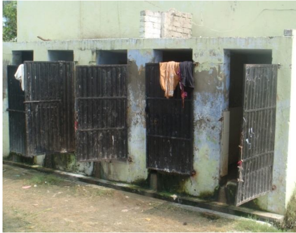
Toilets at the Kandhla Camp
